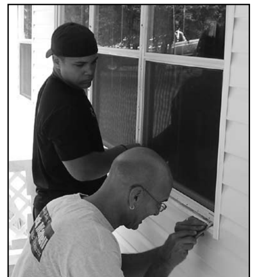
Chris Norton of Grace Church, Keswick, Va., and Doug Marshall-Steele work on repairing windows at a 2007 EAM work camp site.
